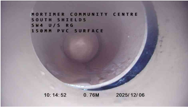
1, 00:00:07, 0.76 m Open joint, large
